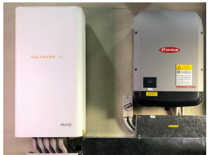
Figure 1: A SolShare installed with a Fronius inverter.
